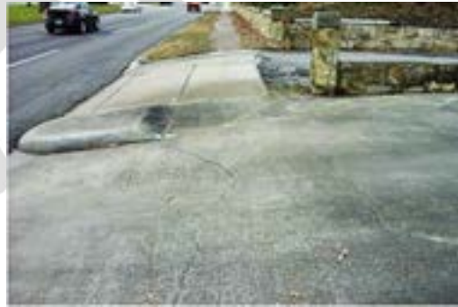
Non-compliant cross slope
