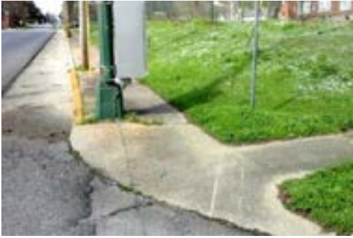
Obstruction with utility box
