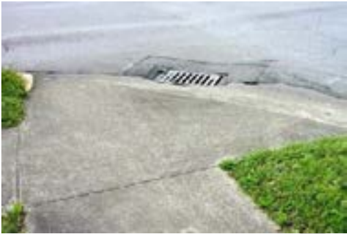
Storm drain blocking ramp
