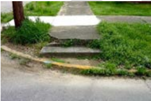
Missing ramp - steps
