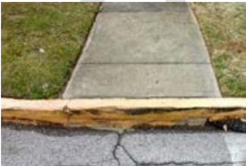
Missing ramp – curb
